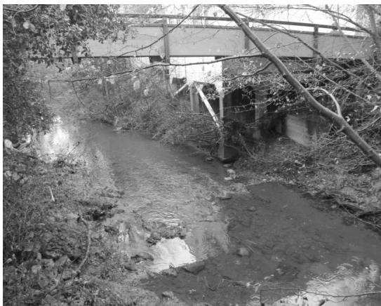
San Anselmo Creek is a popular gathering place and viewing area, but overflowing banks generated damaging floods during winter storms on several occasions.
