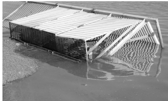
Pumps and a tidal gate on the levee east of Shorebird Marsh control tidal and stormwater flow into the marsh. High tides overwhelming this structure are a portent of impacts from rising seas to come.
